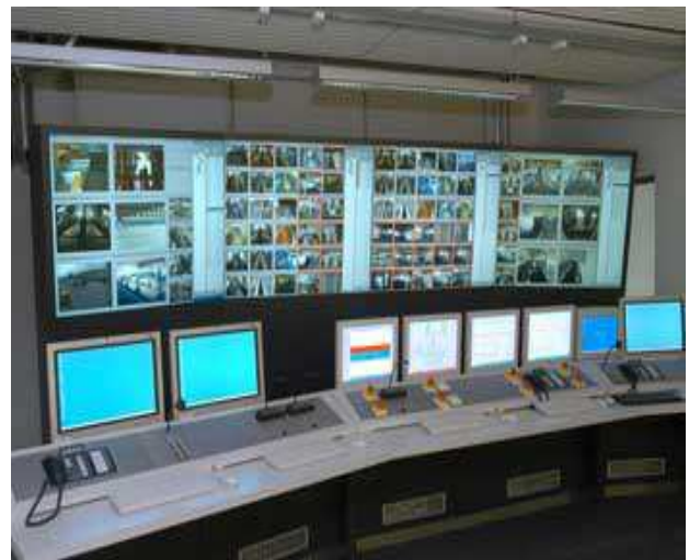
Fig. 1. Central Control Room scheduler Computers (CCR IKCO's)
